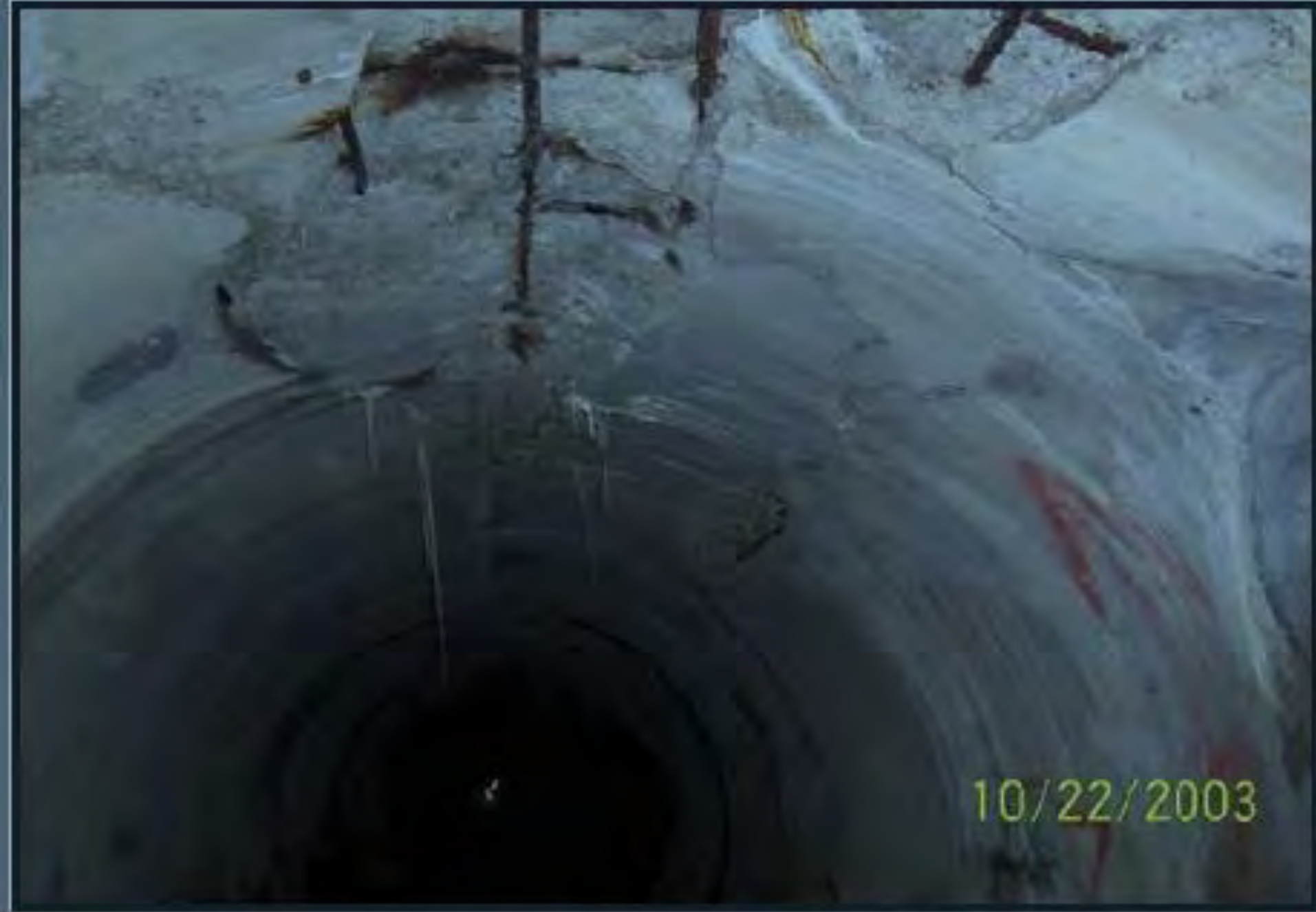
CRACKED AND CORRODED RIGID SEWER PIPE
